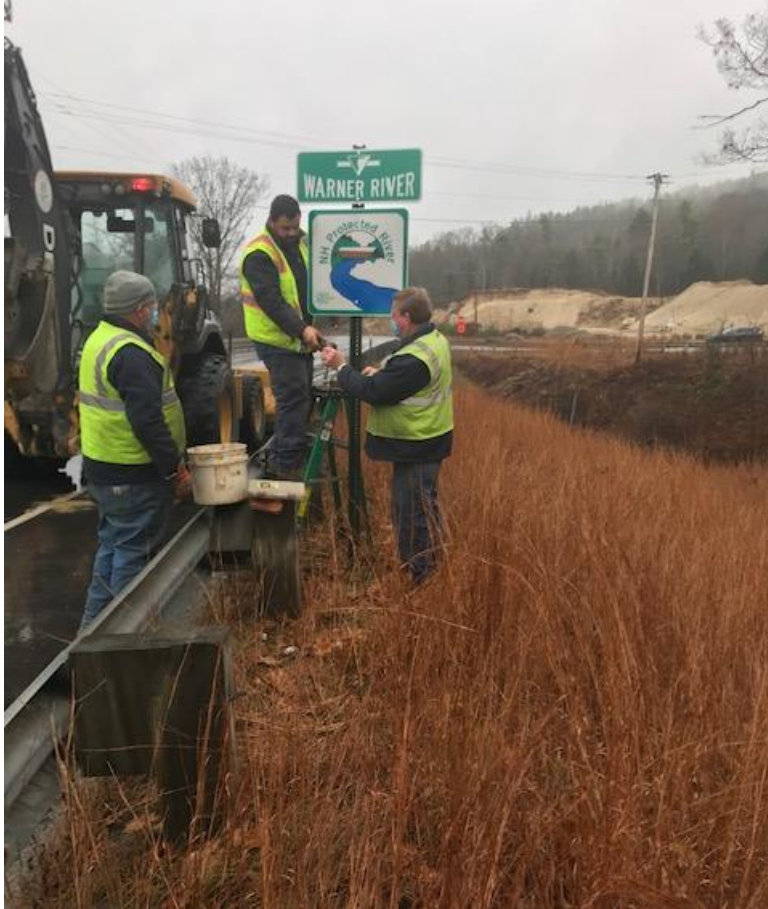
Steve Hall, Justin Fitzgerald and Rick Churchill installing a protected river sign. Photo by Scott MacLean
