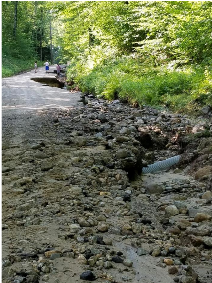
Cressy Road Washout
