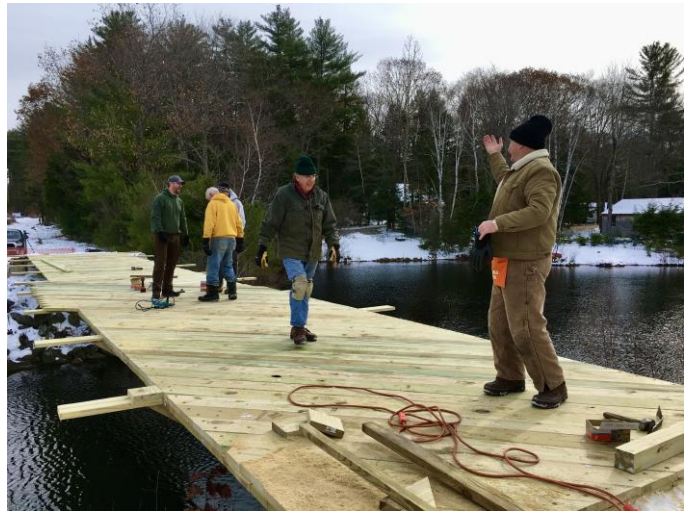
Robert D. Saturley Bridge an architecturally consistent Americans with Disabilities (ADA) entrance.
